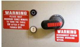
Power Panel (behind table)
