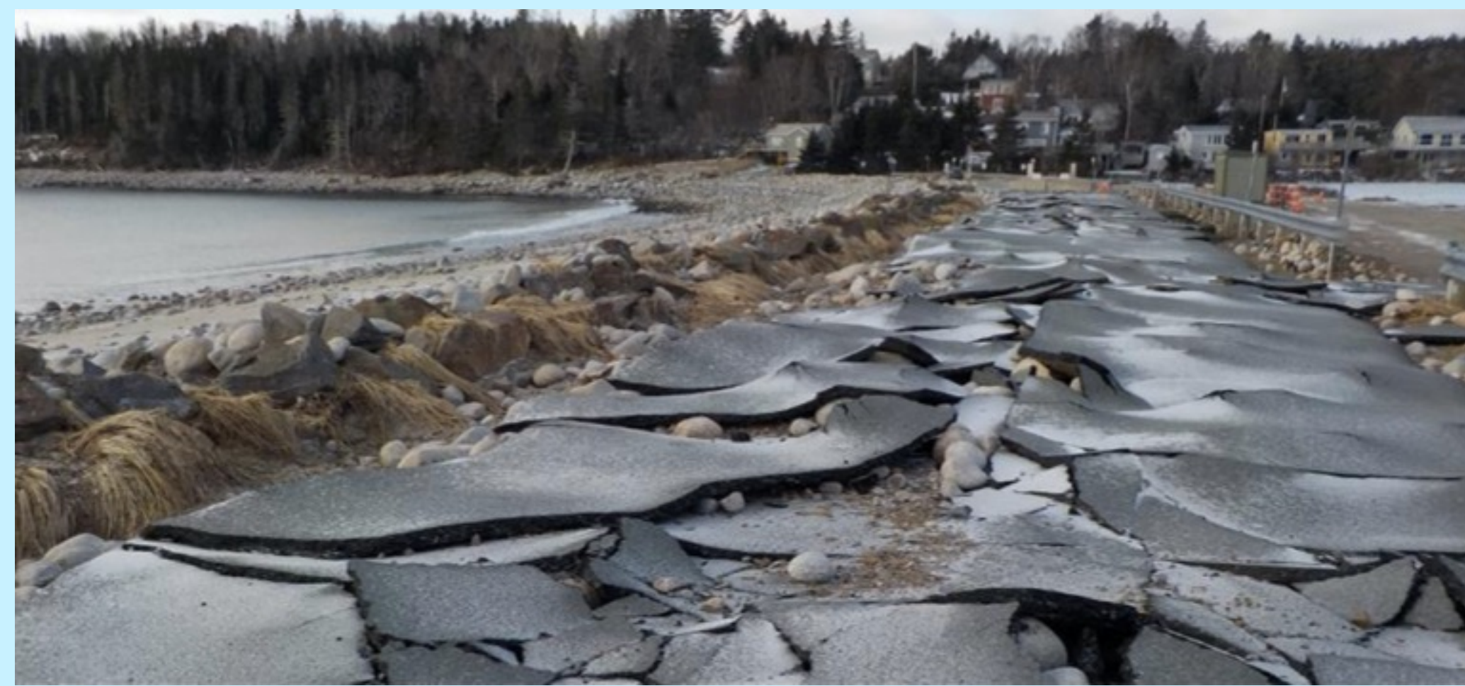
Figure 1. January 2018 winter damage to Conrads Road.
