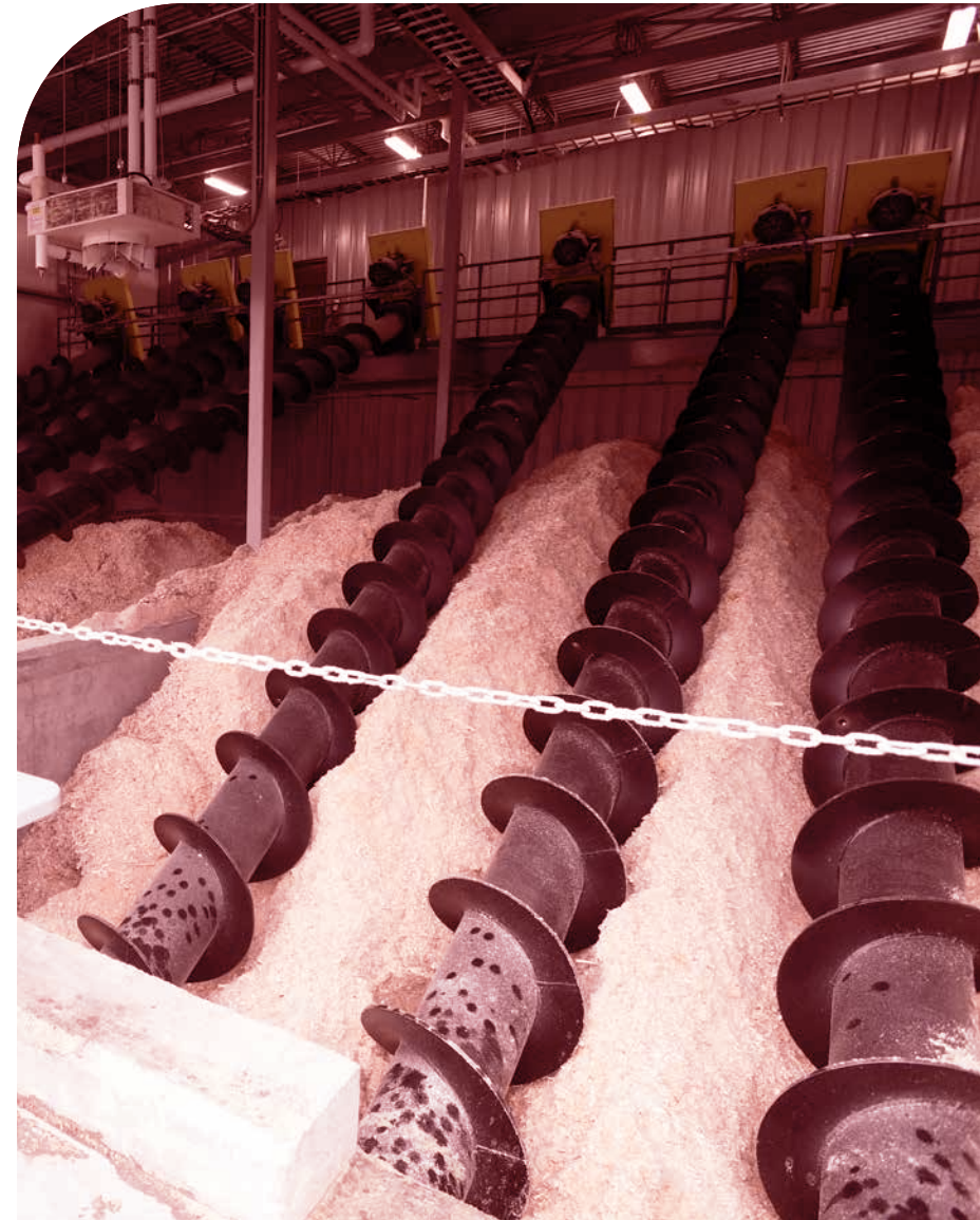
Agricultural Campus biomass cogeneration plant
