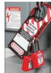
Panel and breaker locks
