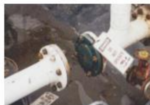
Pipe Blinding Flange
