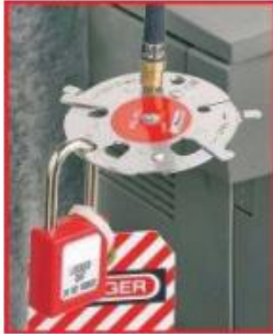
Locked Comp. Air Line
